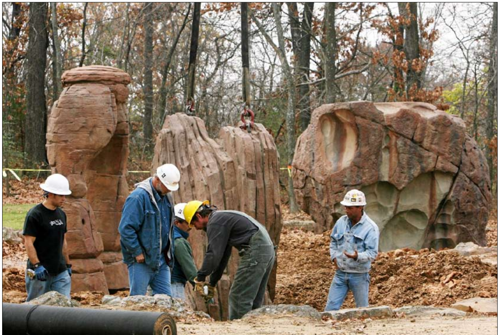
Workers install three new rock climbing boulders near the entrance of Turkey Mountain on Monday. Photos by JAMES GIBBARD/Tulsa World
